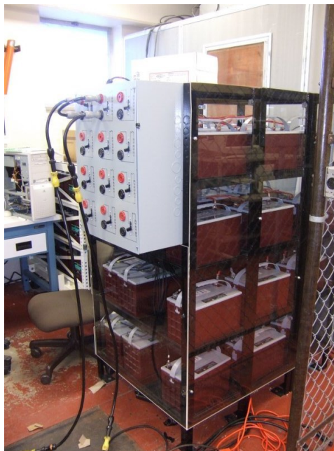
Figure 5.10: The load bank power storage array.
