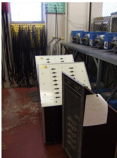
Figure 5.9: The static load banks.
